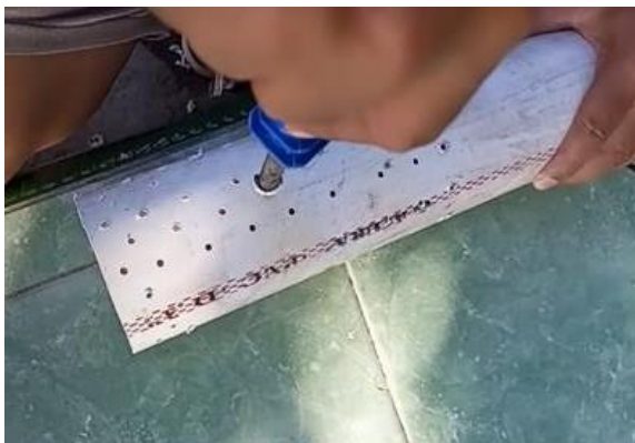
Figure 1. PVC Pipe Perforation
