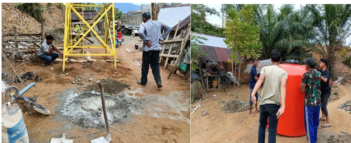
Figure 2. Community-based WASH infrastructure developed to improve access to safe water and hygiene facilities in flood-affected rural communities.
